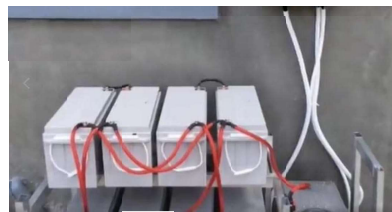
备用电源 Backup Power
